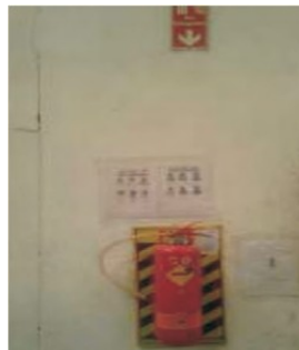
Fig. 6.7.1.1: Extinguisher kept in the wall with necessary identification
